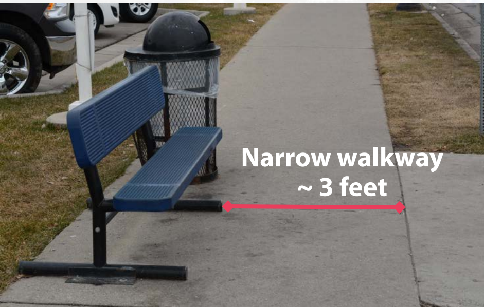
Missing sidewalks on 300 W
